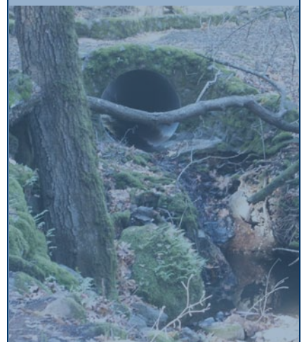
The stone faced culvert on the hiking and equestrian trail between the Zezza and Kerrigan properties.
